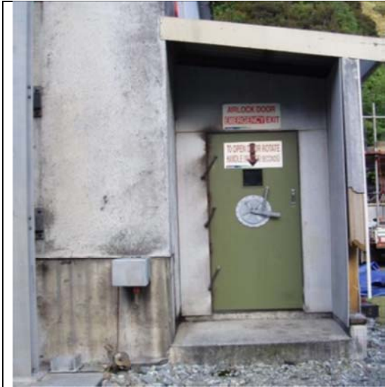
Picture 1: Airlock room outside entrance
