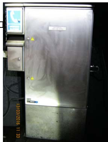
Picture of refuge with telephone, radio and gas detection equipment
