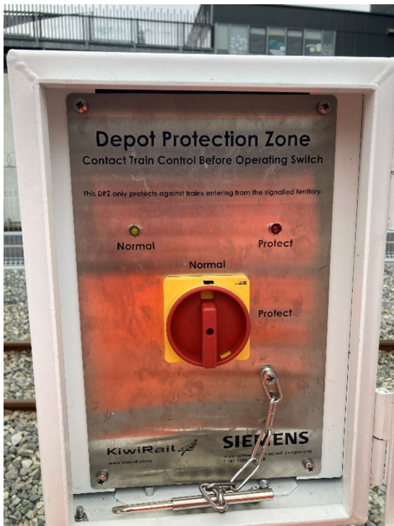
Depot Protection Zone box switch and lights
