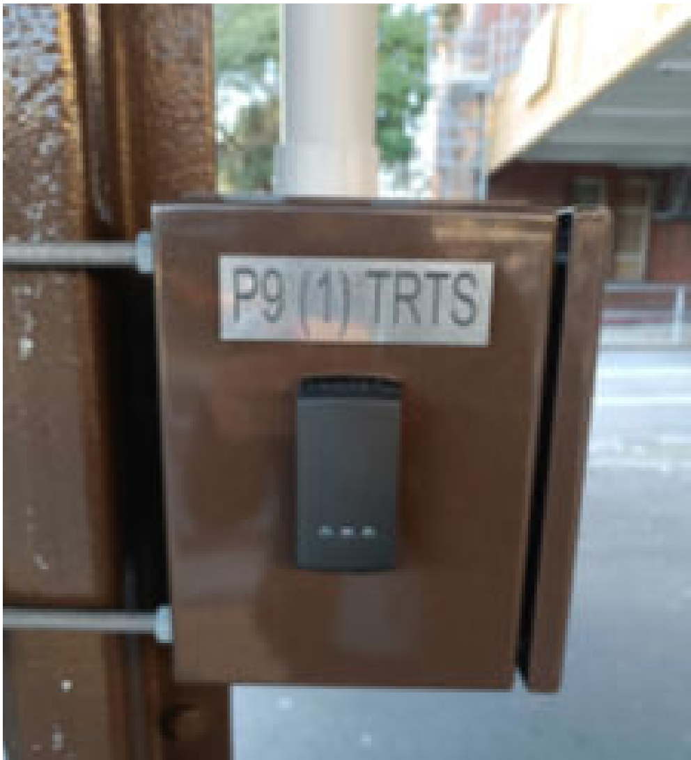
TRTS panel label and RFID reader
