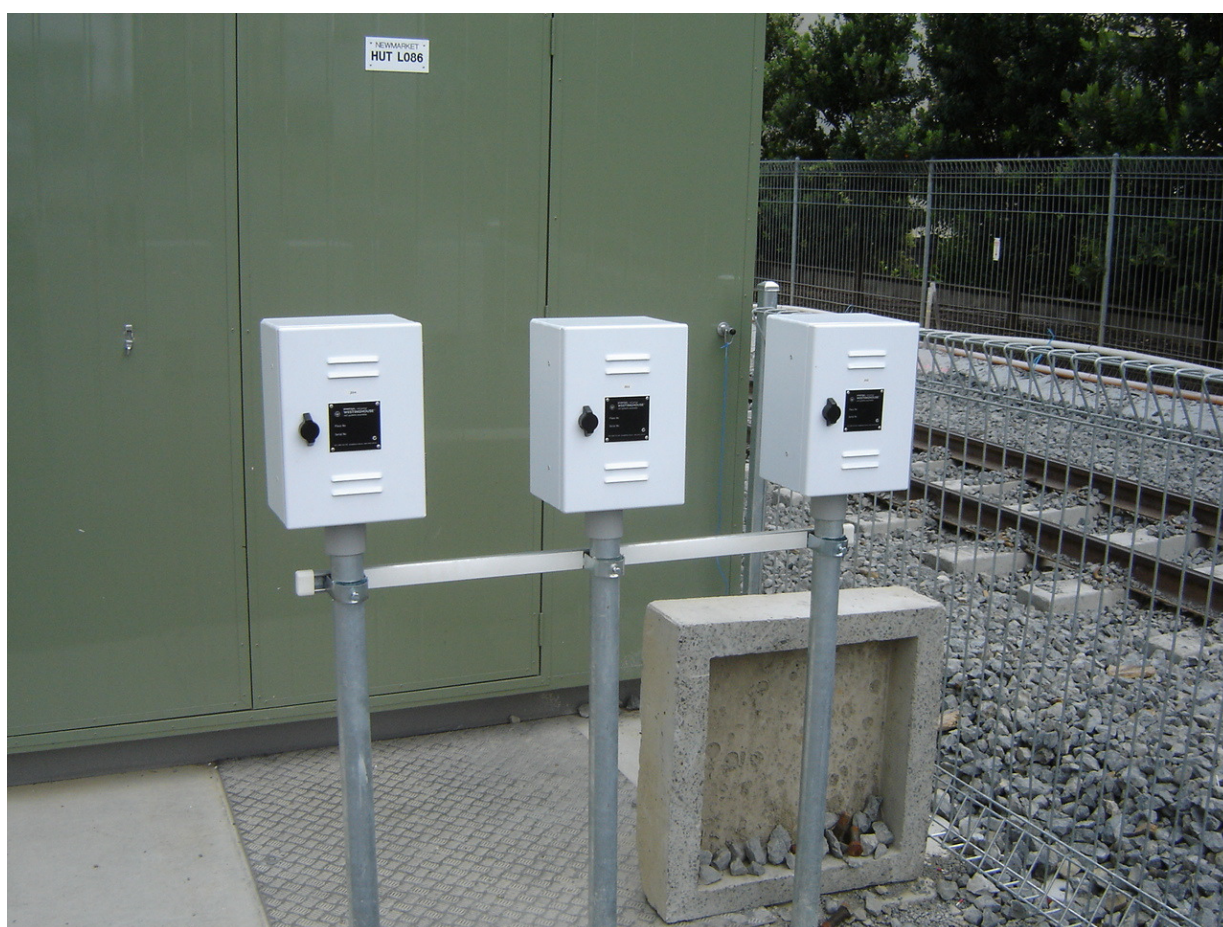
Example of Lockout Control Boxes
