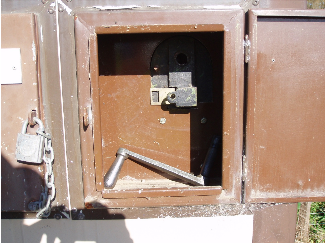
Picture showing crank handle in the bottom of the location box, but not in the detection holder.
