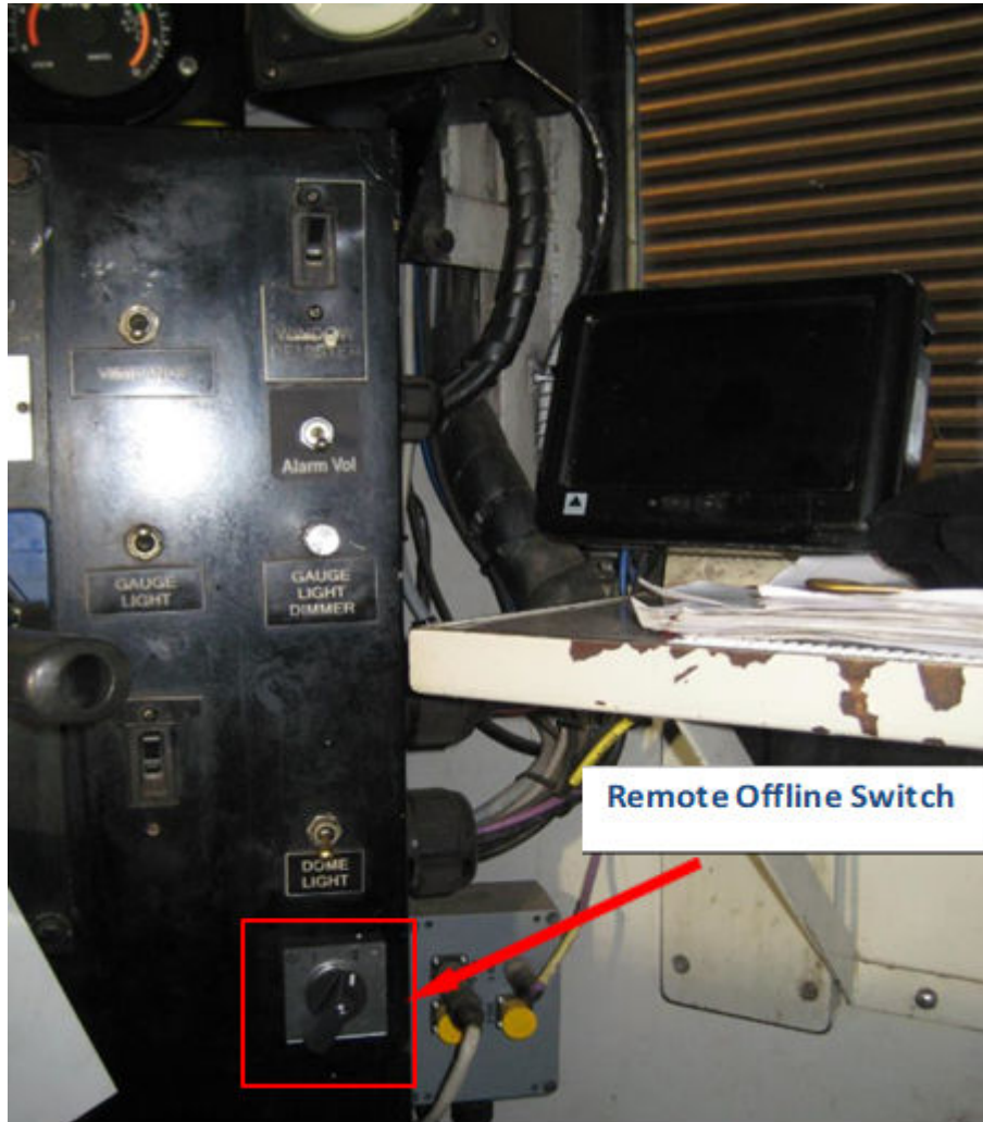
Remote Offline Switch Location
