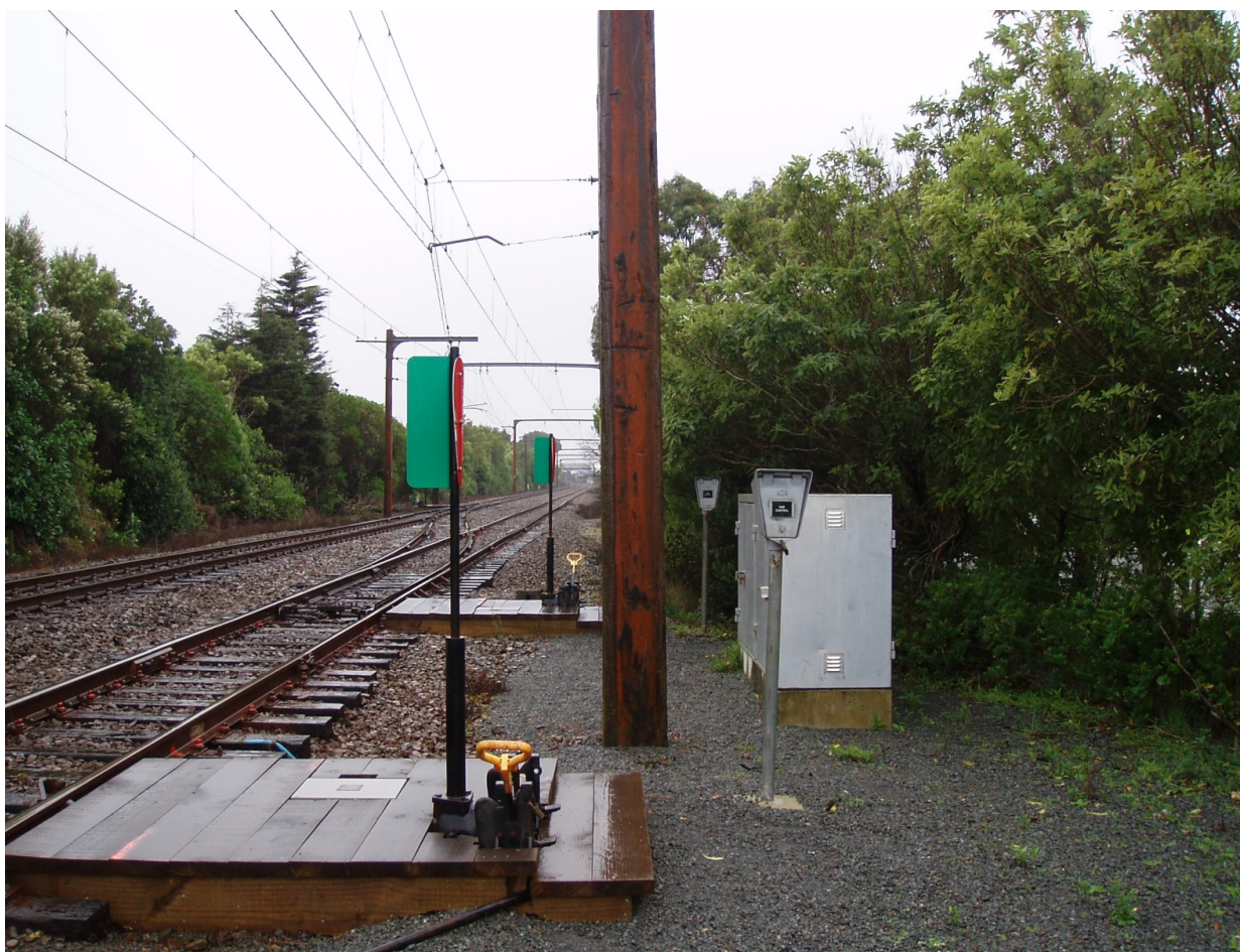
Picture 1: Woburn North Siding showing location of points lock control boxes adjacent to the Down main.
