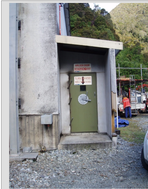
Picture 1: Airlock room outside entrance
