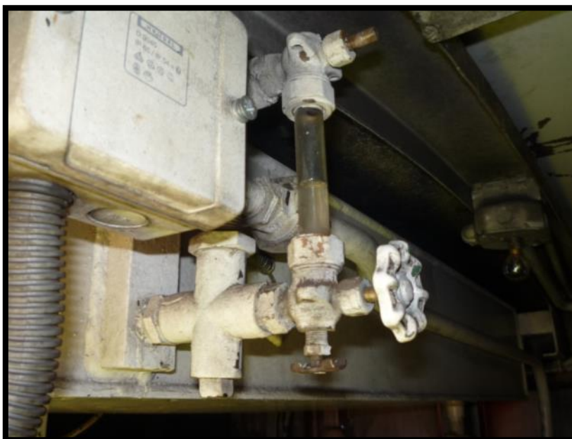
Figure 10: Header Tank and Water Sight Glass
