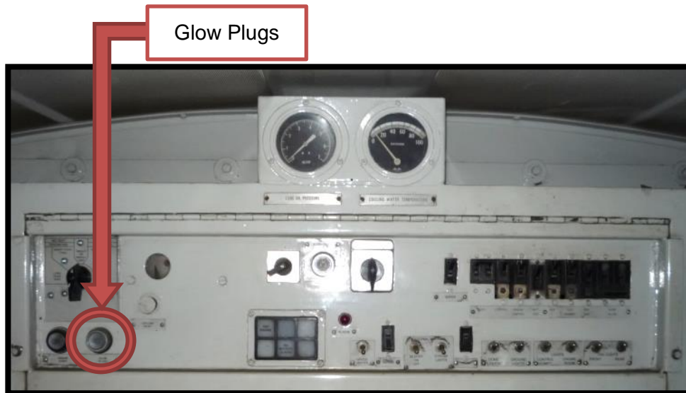
Figure 26: Cab Electrical Board
