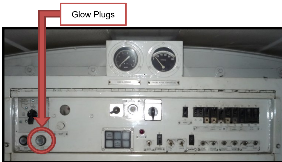
Figure 26: Cab Electrical Board
