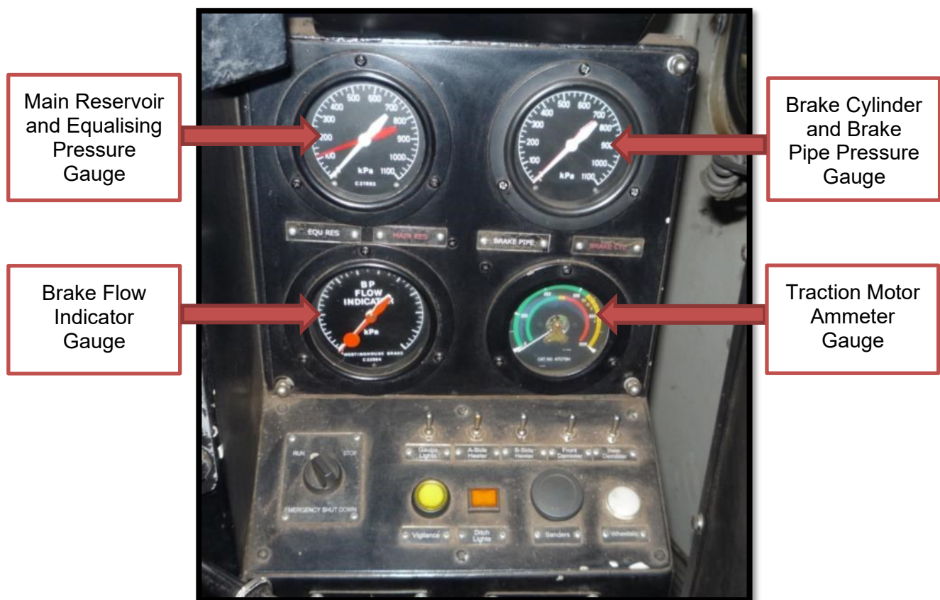
Figure 12: Control Stand Gauges
