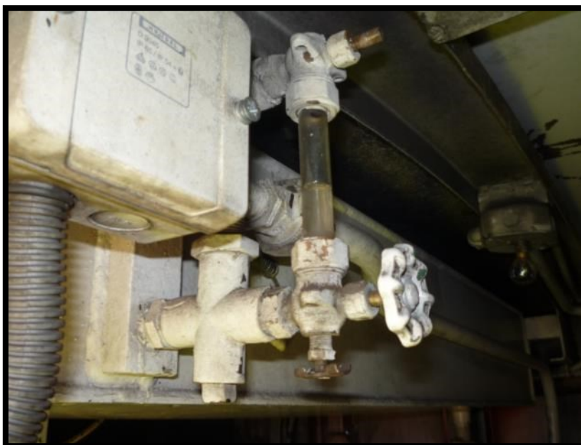
Figure 10: Header Tank and Water Sight Glass
