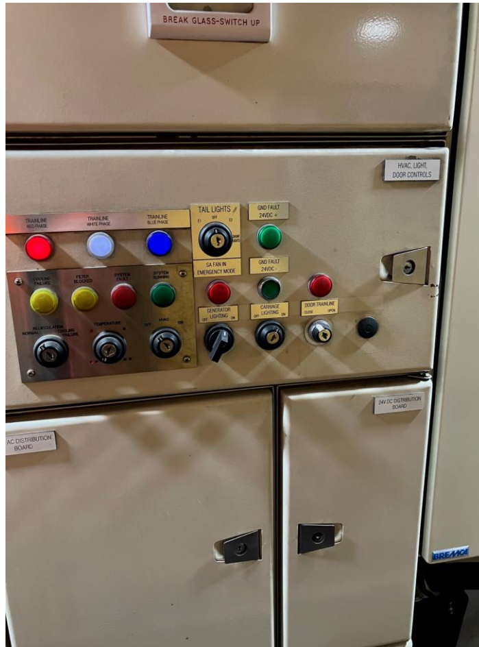
Generator room lighting and air conditioning controls
