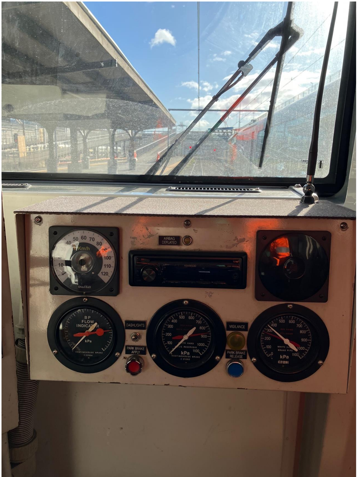
SRG gauge panel controls, indicators, and gauges
