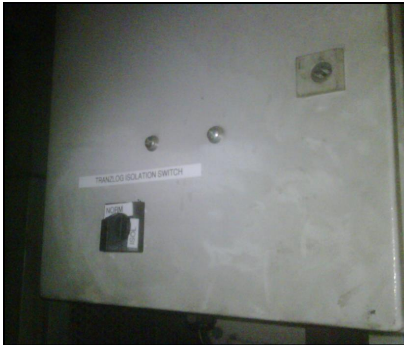
Figure 54: Tranzlog Isolation Switch
