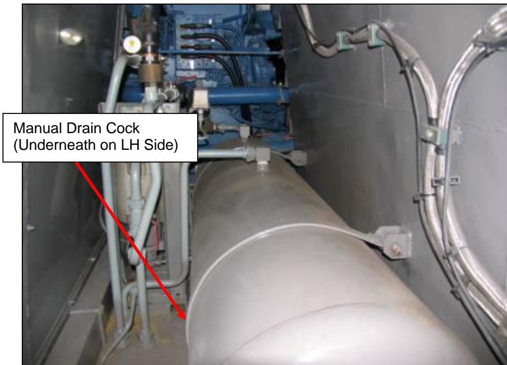
Figure 29: No.2 Main Reservoir
