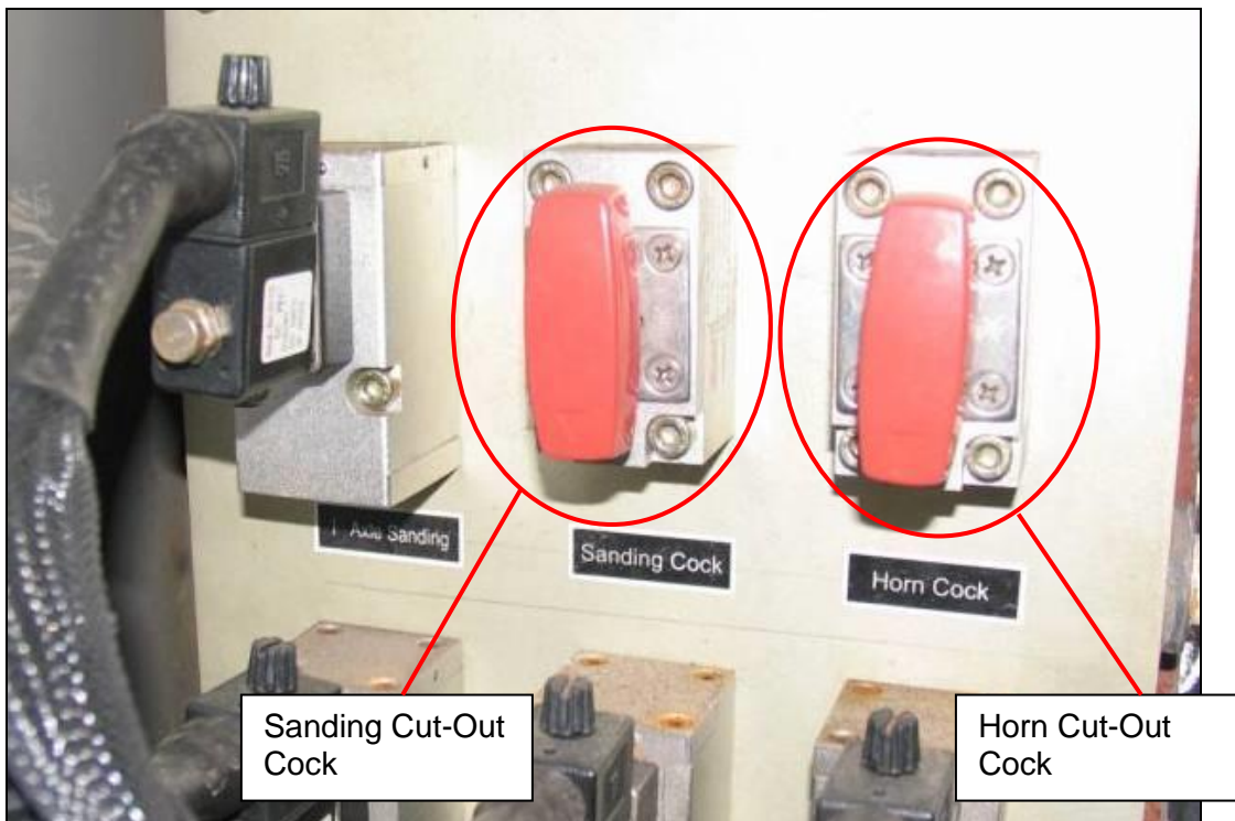
Figure 60: Pneumatic Control Manifold No.2 End (In radiator cabinet)
