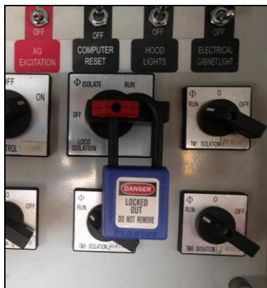
Isolation Switch – OFF
