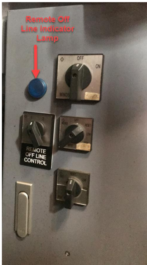
Figure 8: Driver Console Right Under Desk Switches
