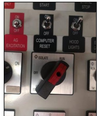
Isolation Switch - RUN
