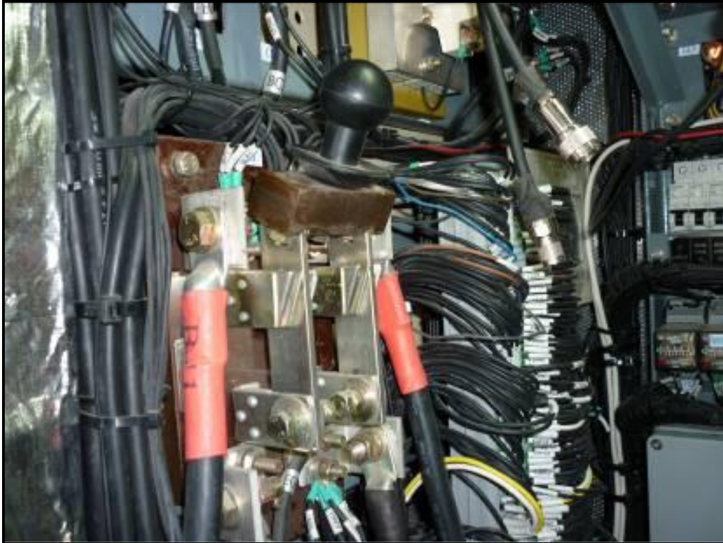
Figure 34: Battery Knife Switch
