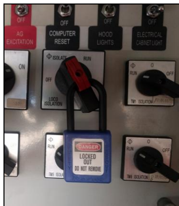
Isolation Switch - ISOLATE
