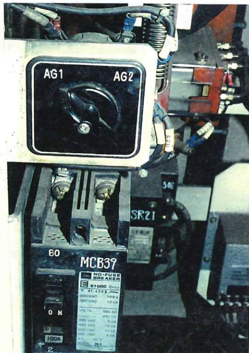
APCOS in No.2 End Control Cabinet
