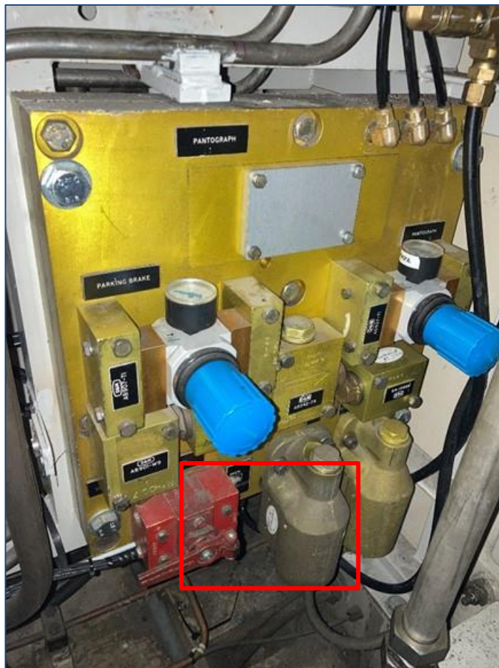
Fig. 16 Manifold 2 Control Reservoir cut out valve.
