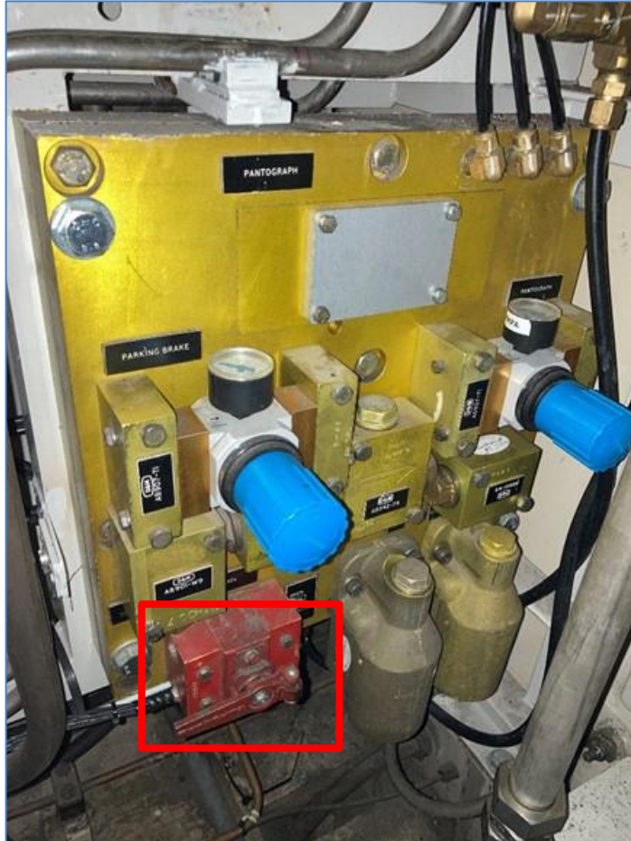
Fig. 12 Control reservoir cut out valve.
