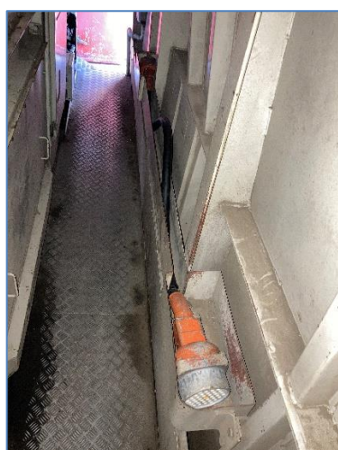
Fig.6 Jumper cable storage
