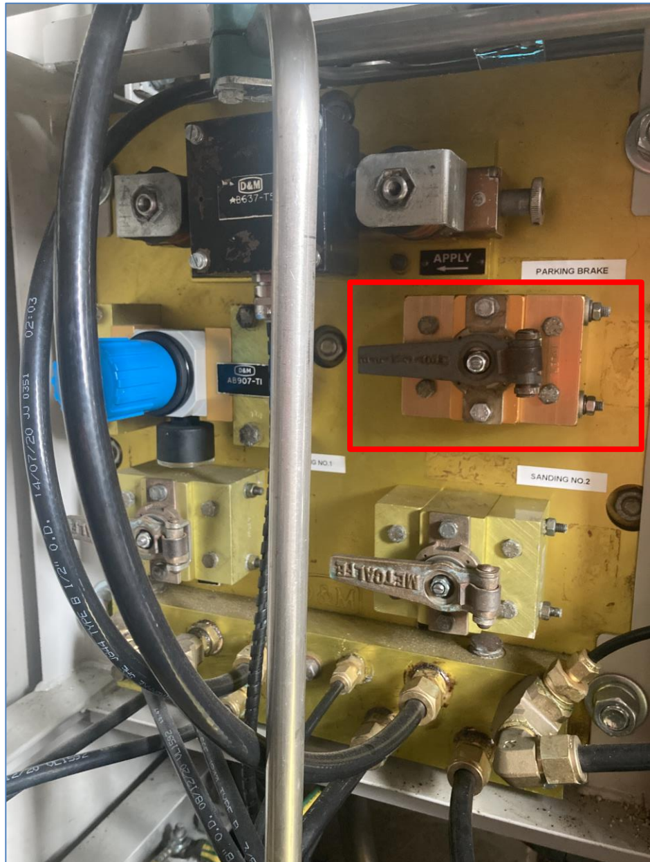
Fig. 10 Brake rack isolation valve for the Park Brake
