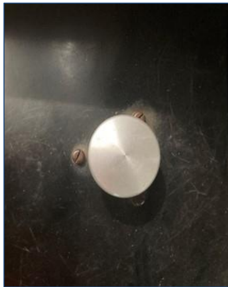
Fig. 35 Assistant Emergency Stop pushbutton
