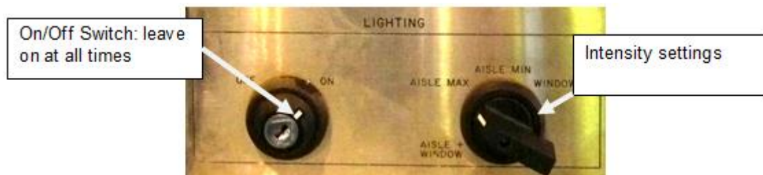
Figure 20: Lighting panel - AK switchboard.
