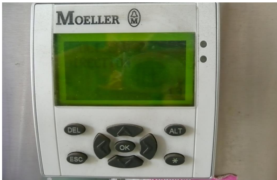
Figure 46: Train management control panel.
