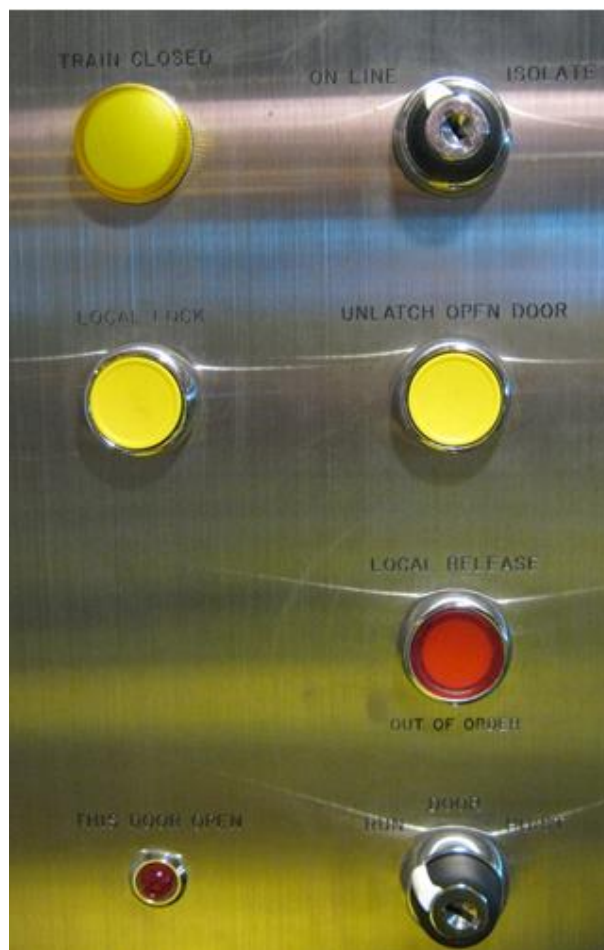
Figure 52: Wheelchair hoist control panel.
