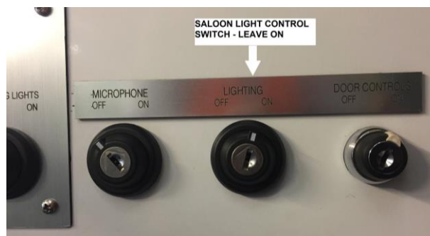
Figure 21: Lighting panel - AKS switchboard.
