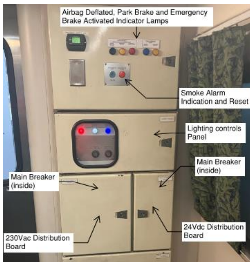
Figure 4: AKS electrical control cabinet
