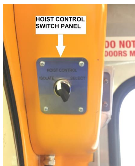
Figure 53: AKS Hoist Control Panel.
