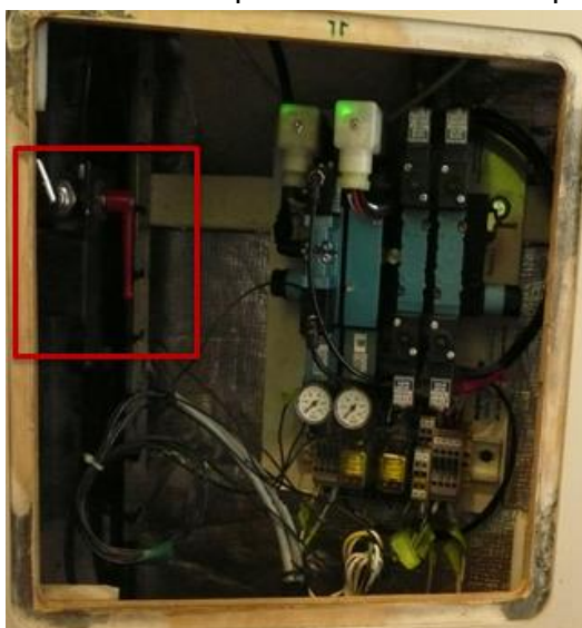
Figure 31: Door and step isolation cocks
