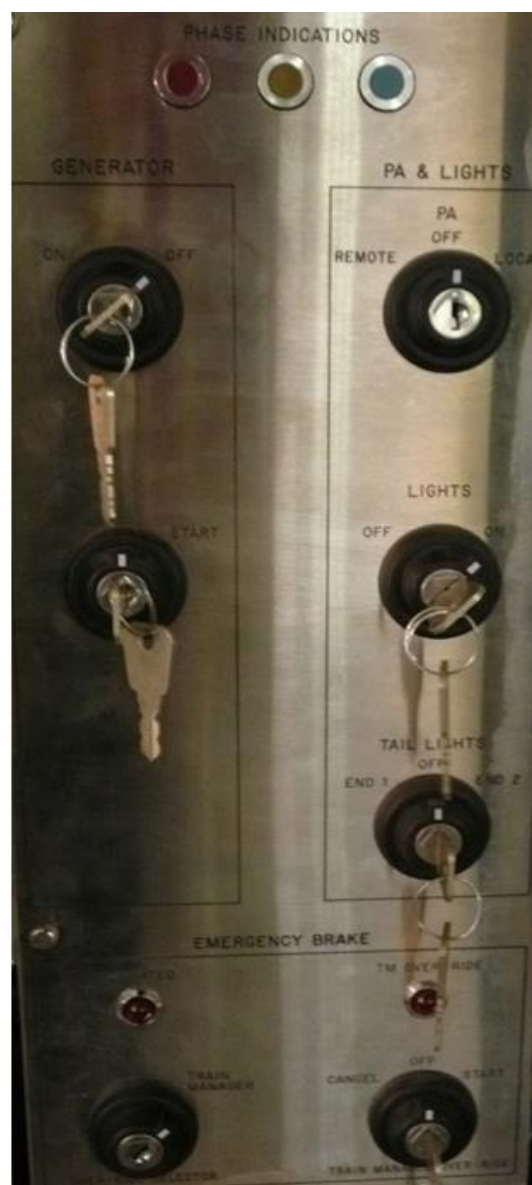
Figure 2: AKV control panel
