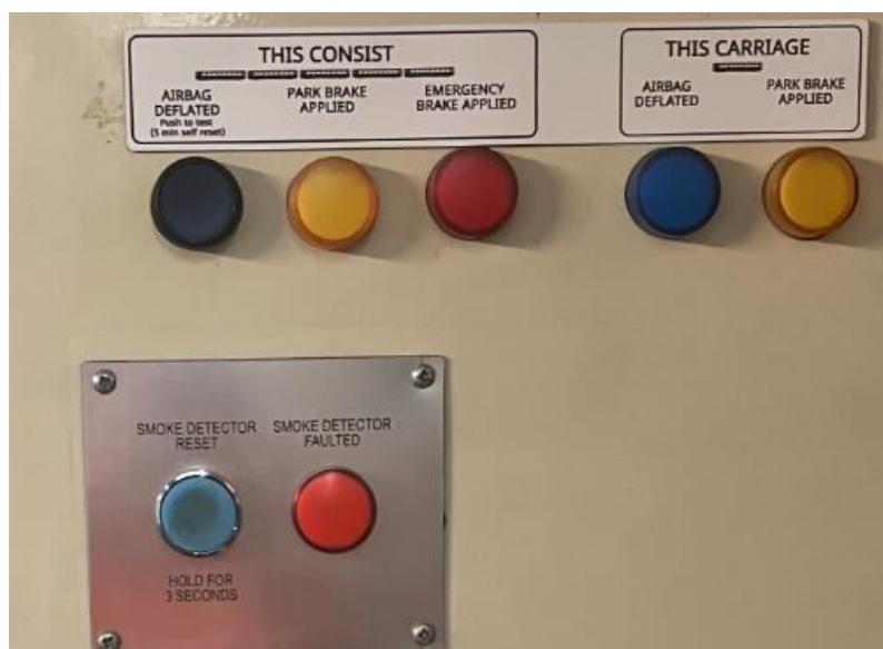
Figure 45: AKS TMS Alarm Panel
